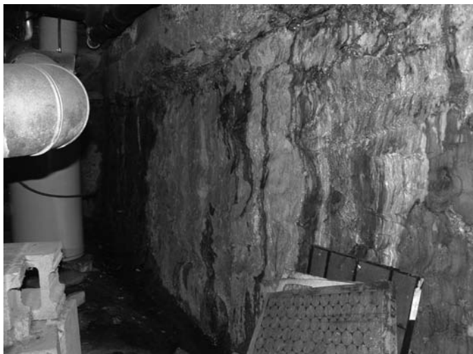
A basement in Vermont with severe mold problems – a known asthma trigger. Mold removal was a common housing intervention in both Boston and Vermont.
